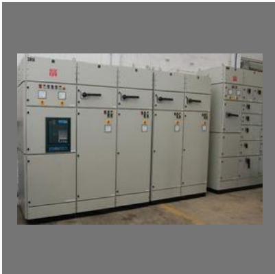
Electric Control Panel
