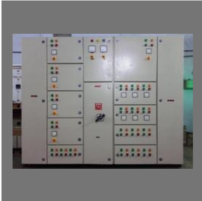
Crushing Plant Panel
