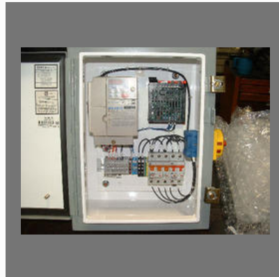
DC Drive Control Panel
