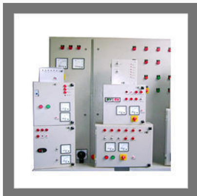
Electrical Control Panel Board
