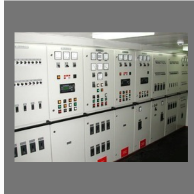
Electrical Power Panel
