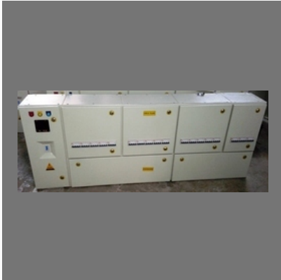
Power Distribution Panel
