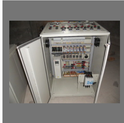
AC Drive Control Panel
